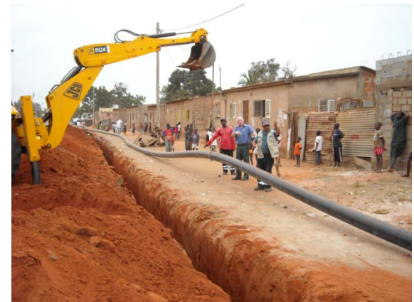
Angola, Luanda Water distribution System
